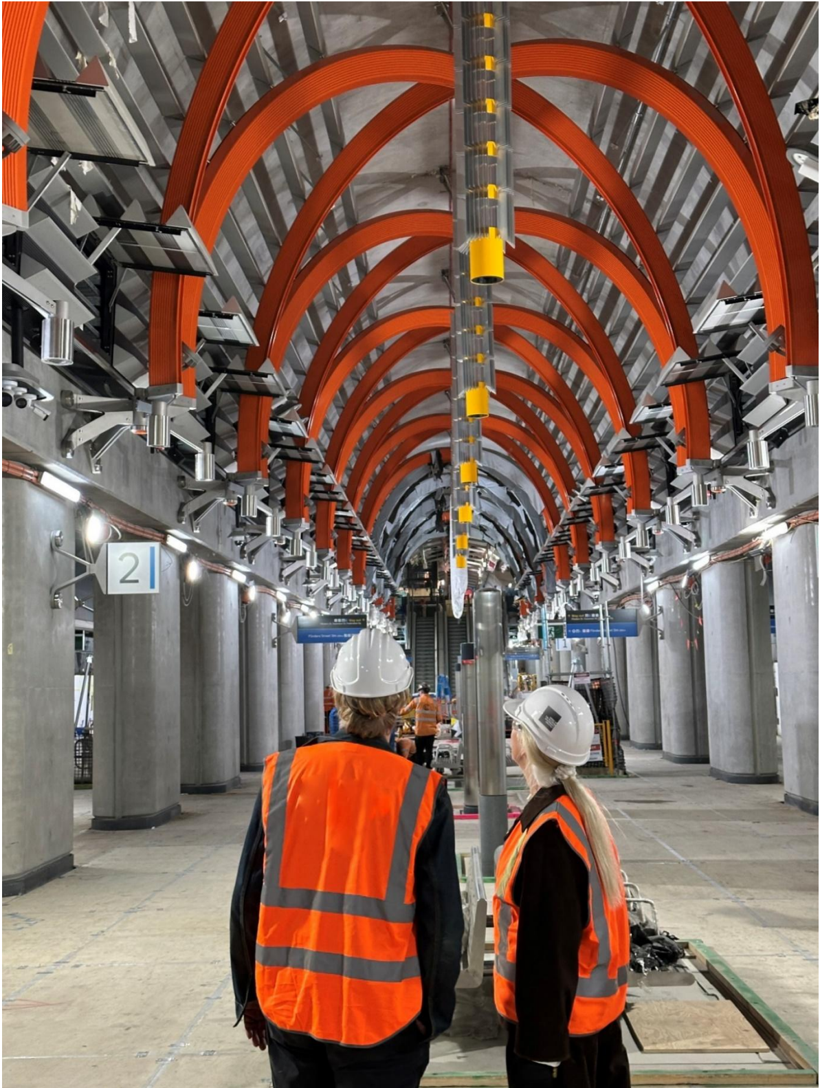
Metro Tunnel Project, Melbourne / Wurundjeri Woi-wurrung Country (In delivery, opening late 2025) Architecture: Collaboration with Hassell, Weston Williamson and Partners and Rogers Stirk Harbour and Partners Photography: OVGA Client: Metro Tunnel Project OVGA role: Strategic advice, tender evaluation and design review during project planning, procurement and delivery.
